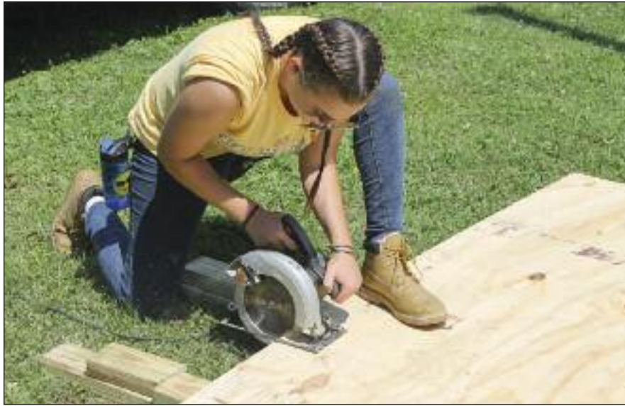
A teen works with a circular saw on her work site in Harlan, Kentucky.
